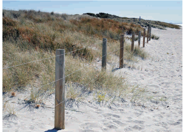
Half round or small round treated posts with two or three galvanised wires strained between accessways is the most common method of fencing along the toe of foredunes to protect native sand binding vegetation including new plantings.
